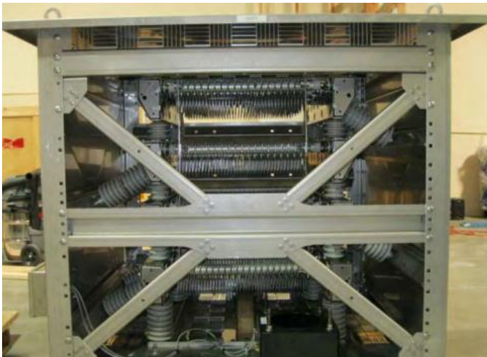
View of low resistance grounding enclosure bracing and additional resistor assembly supports.
